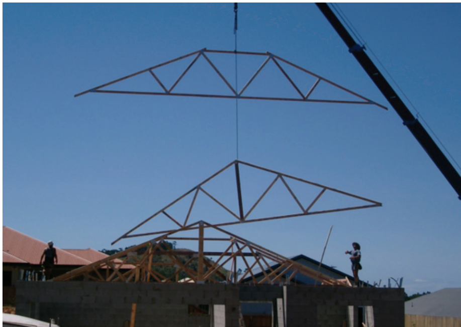
Photograph 3 – Incorrect lifting of trusses
