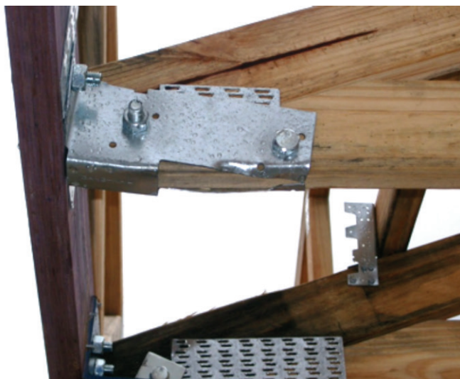
Photograph 7 – Girder brackets not installed correctly
