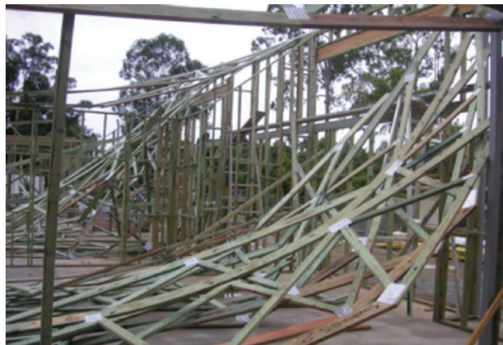
Photograph 4 – Dangers of not providing temporary bracing
