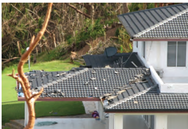
Photograph 3 – Inadequately fixed tiles dislodged after high wind event
