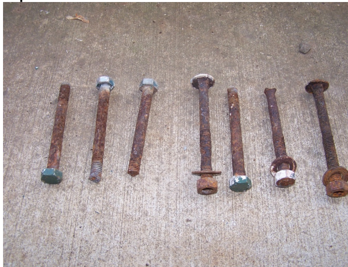
Severe corrosion of bolts removed from deck bearer to post connections
